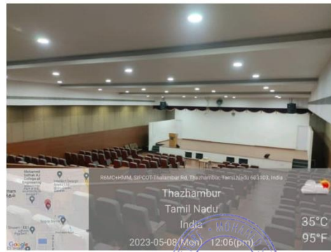
LED LIGHTS @ AUDITORIUM
